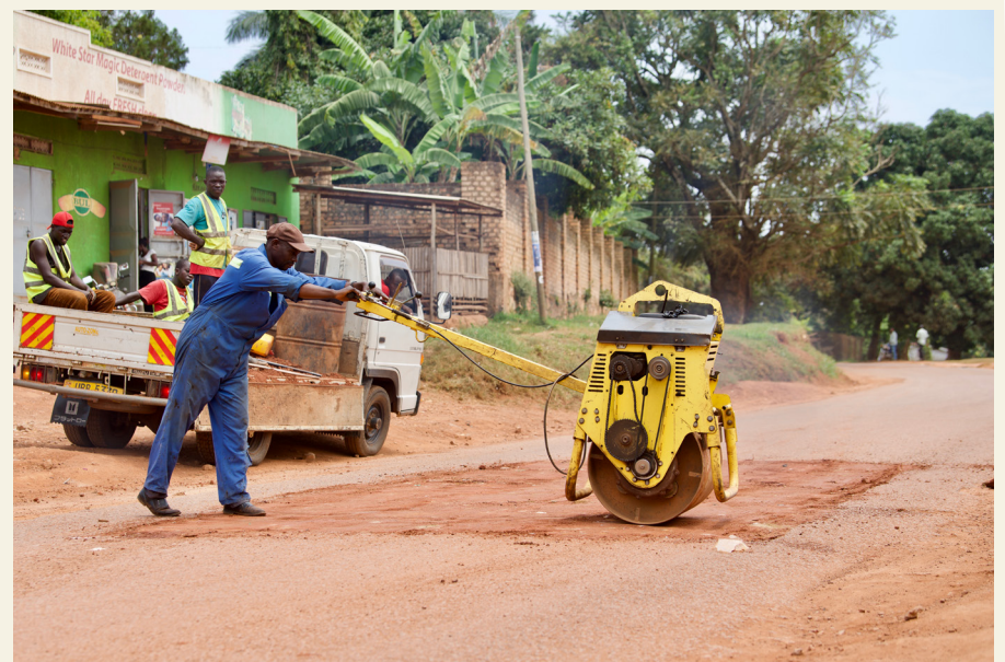
A worker filling up a pothole on a road in Kampala. The 2018 Africa infrastructure development index puts Uganda at the 27th position out of 53 countries
