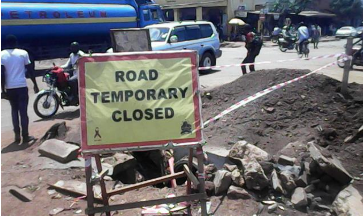
Photograph 4: Caution message placed at the exact point where the road was closed along Jinja Main Street, Jinja Municipality – Eastern Region
